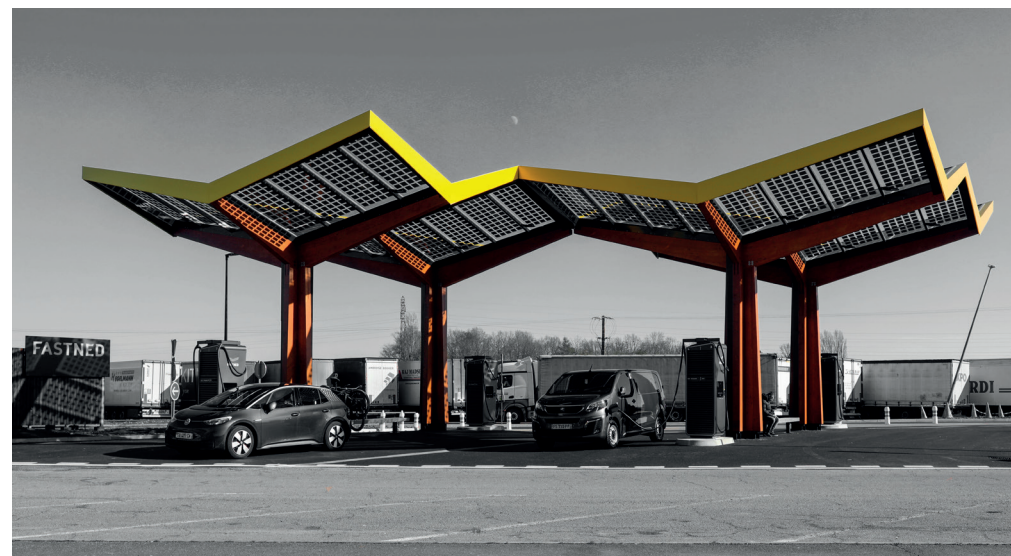
High-Power electric charging stations installed by Fastned at Saint-Ambreuil (Drôme) on the APRR-AREA motorway network
